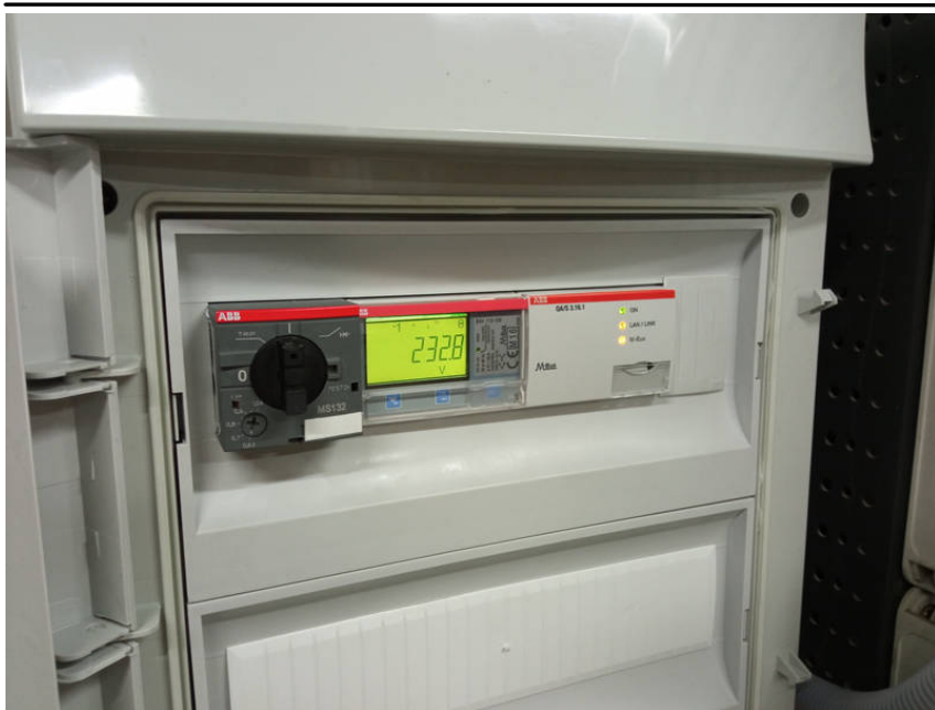
Figure 1. Energy meter with the possibility of remote reading
